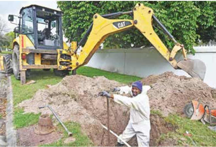
Put a plug in it: City maintenance teams stopping a leak caused by a faulty valve in Onze Molen, Durbanville, late last year.
